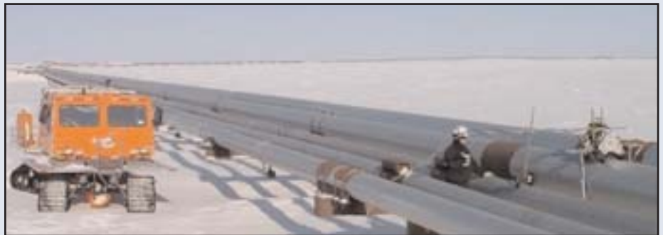
Kakivik Field Lead, Ruel Carlson performing linear array on a 24" line on the North Slope.
